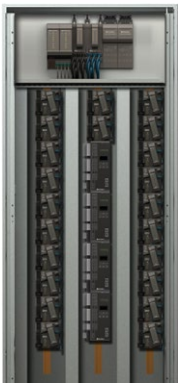
T800 Steam Turbine Digital Electro-Hydraulic Control System (DEH)
